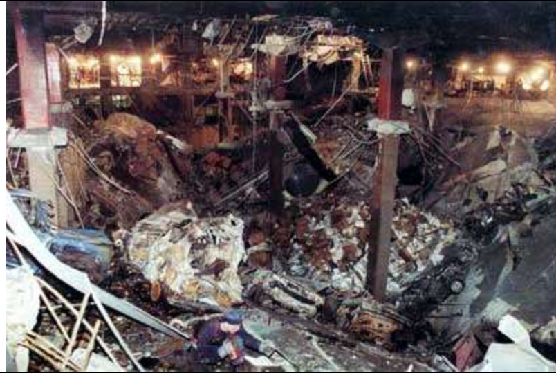
Damage from 1993 World Trade Center Attack
